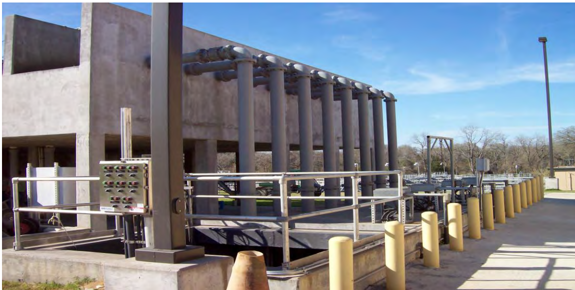
Inlet Lift Station
