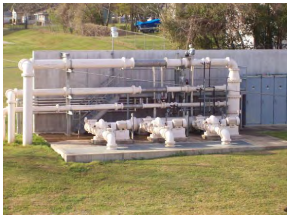
Raw Water Pump Station
