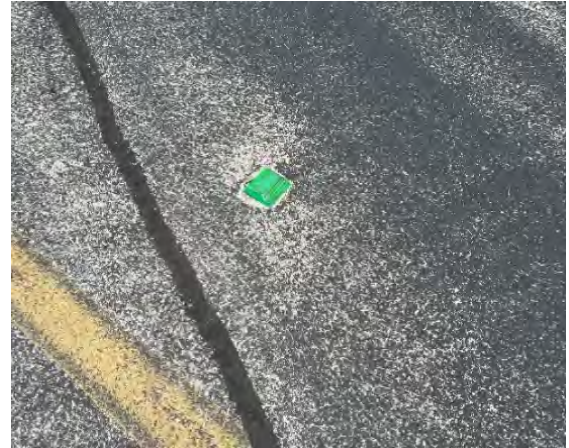
Taxiway Centerline Reflector
