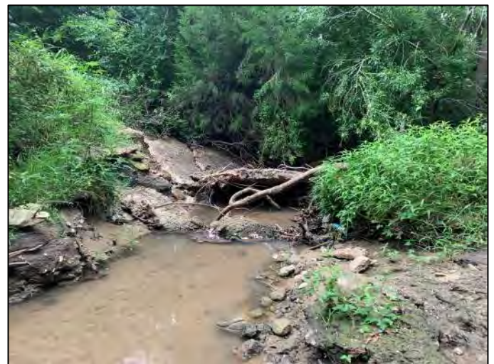
Photo 30: Downstream-facing view of creek and collapsed road.
