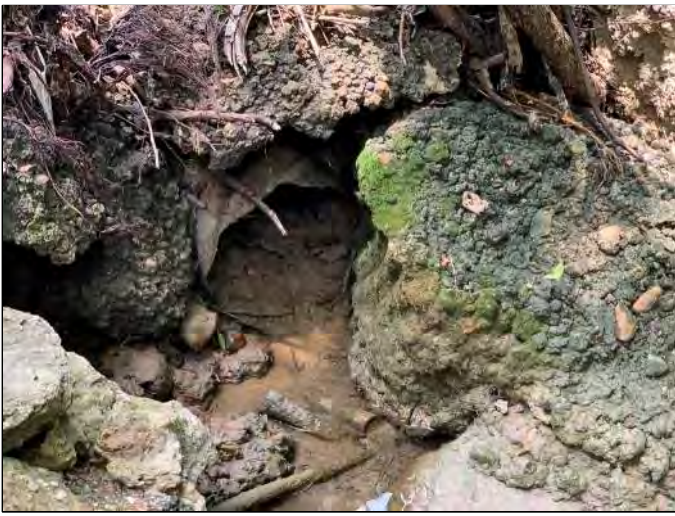
Photo 31: Crushed culvert under collapsed road.
