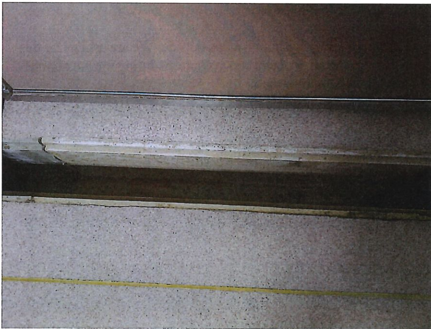
Trough that needs to be covered inside the dog kennels.
