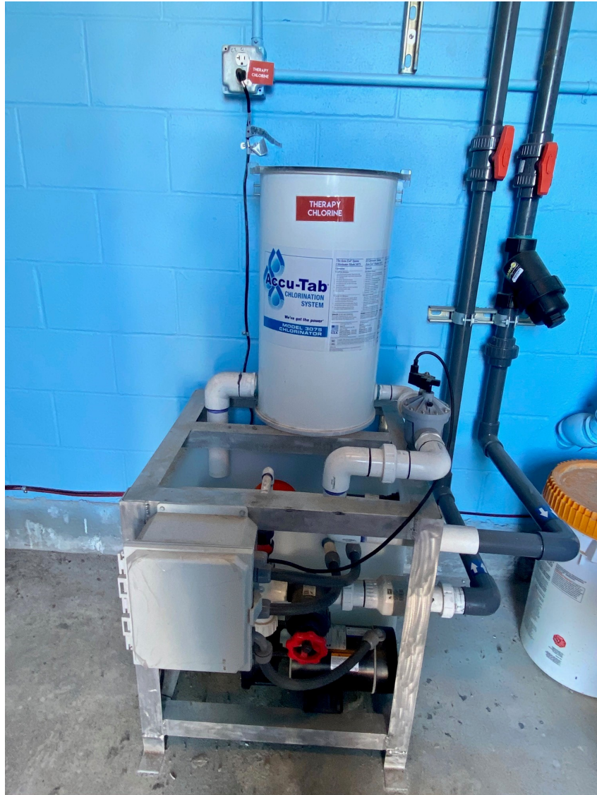
Upgrade to Accu Tab & Acid Rite System - BBAC
