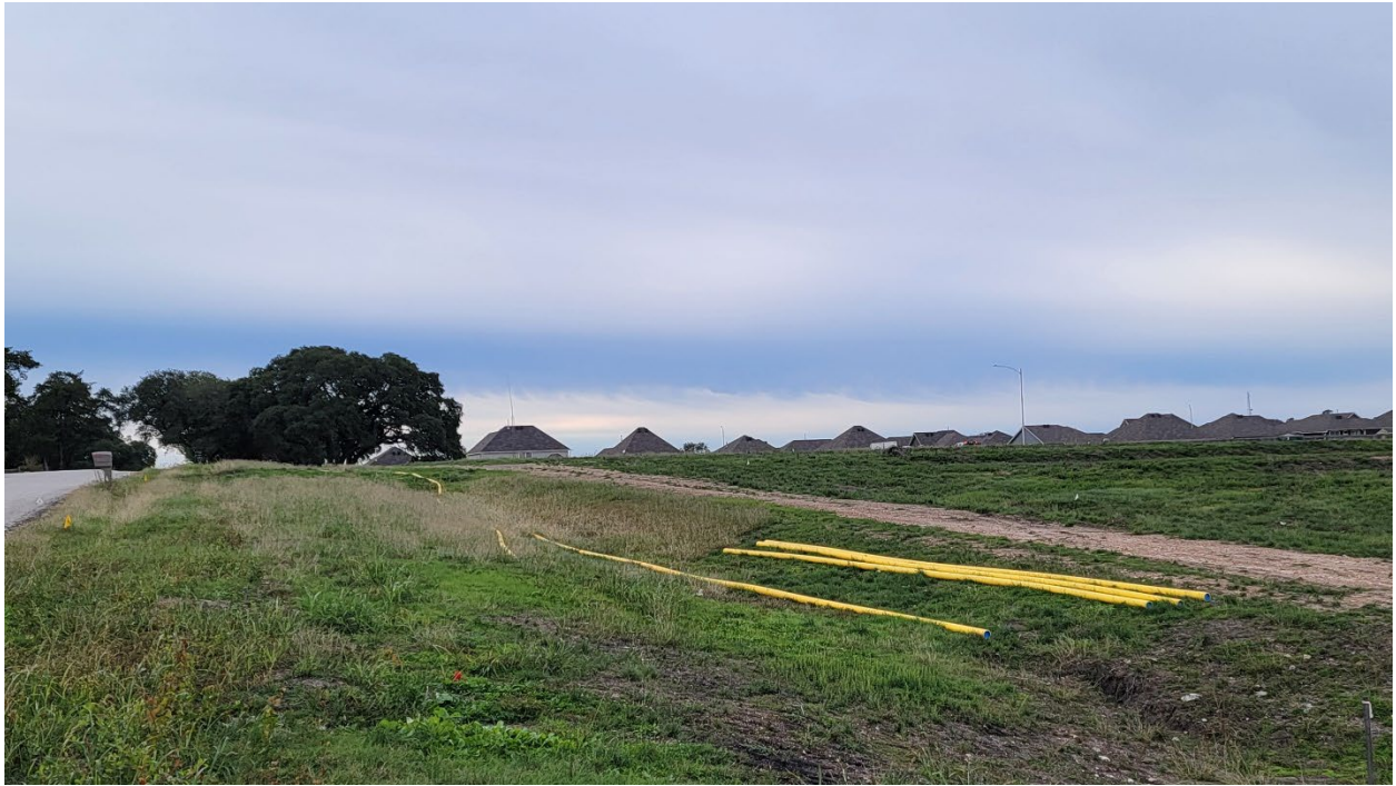
Looking south from Oak Creek Way to the west (Vintage Farms in background. Phase V under construction in foreground
