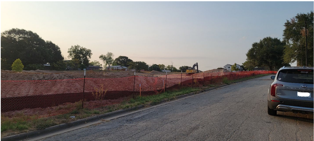
Ebenezer Townhome Development grading work. Adjacent to the south of the subject property. Photo taken on Sabine Street.
