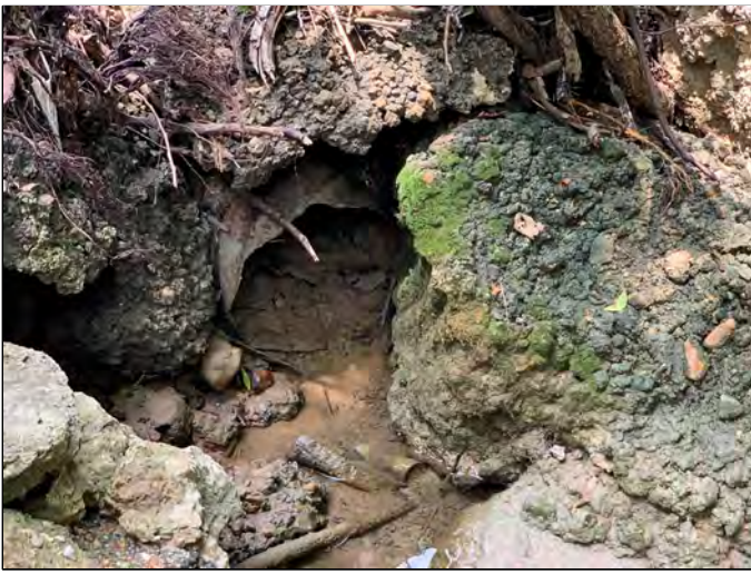
Photo 31: Crushed culvert under collapsed road.
