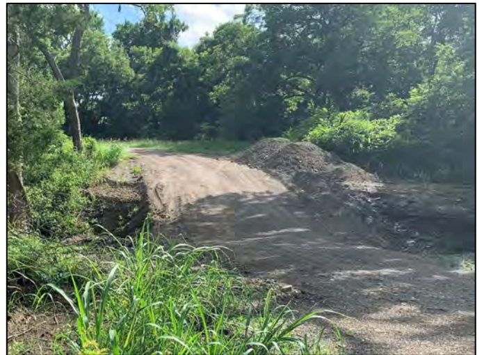
Photo 42: North-facing view of the dirt road crossing the culvert at the southern terminus of the Site.
